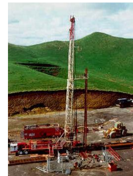
Oil well drilling and water injection
