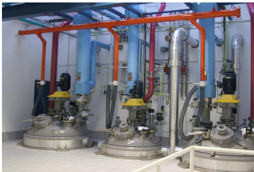
Chemical reactor for the pharmaceutical and biotechnology industry
