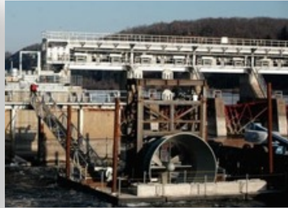
Hydro Green Energy river current turbine
