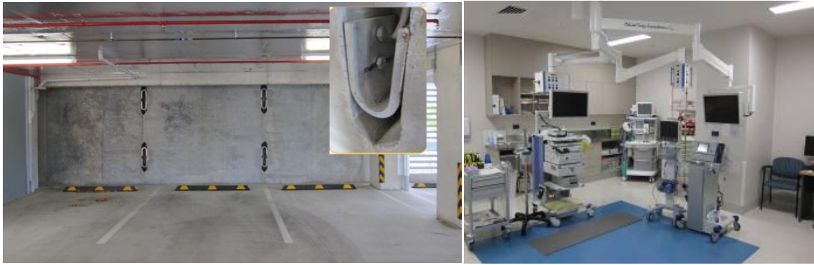
Figure 31: Negligible damage, to both structural and non-structural components, in the Southern Cross Hospital after the earthquake of 22 February.
