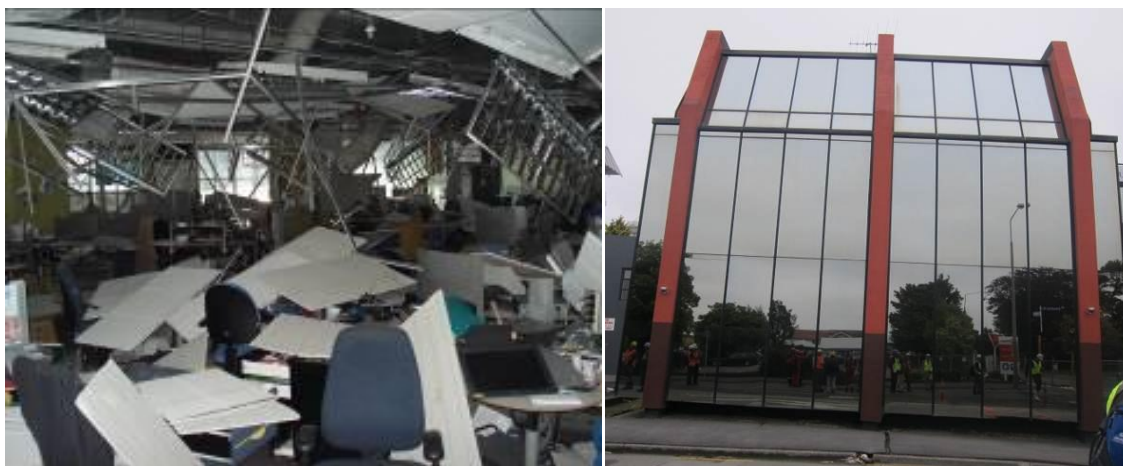
Figure 8: Example of extensive damage to non-structural elements (ceilings and partitions) and of tilting due to differential settlement of the soil-foundation system.
