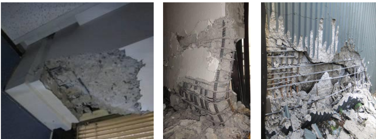
Figure 5: Damage to post-1980s RC moment-resisting frames and walls (Kam et al. 2011, Kam and Pampanin 2011).
