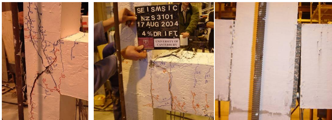
Figure 14: Evolution of seismic resisting connections: performance of beam-column joints designed according to a) pre-1970 codes (shear damage in the joint or soft-storey mechanism); b) capacity design principles as per the NZS3101:1995 (beam plastic hinge) and c) hybrid jointed ductile connections as per Appendix B of NZS3101:2006 (controlled rocking).
