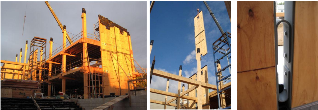
Figure 32: The world first Pres-Lam building implementing unbonded post-tensioned rocking/dissipative timber walls. Nelson Marlborough Institute of Technology, (NMIT), New Zealand (Structural Engineers Aurecon, Devereux et al. , 2011, Architects Irving-Smith-Jack).
